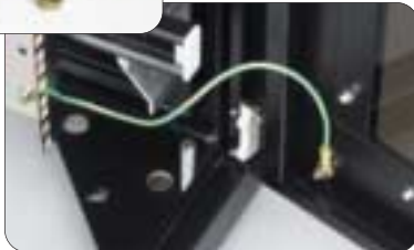
Installed grounding wire kit
