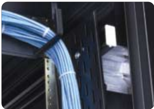
Installed vertical cable tray
